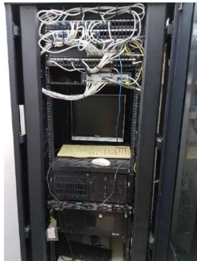
DELL server for programming and testing
