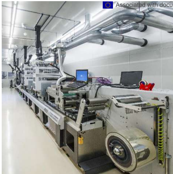
Gallus printing press used in the TEG production process at Innovation Lab
